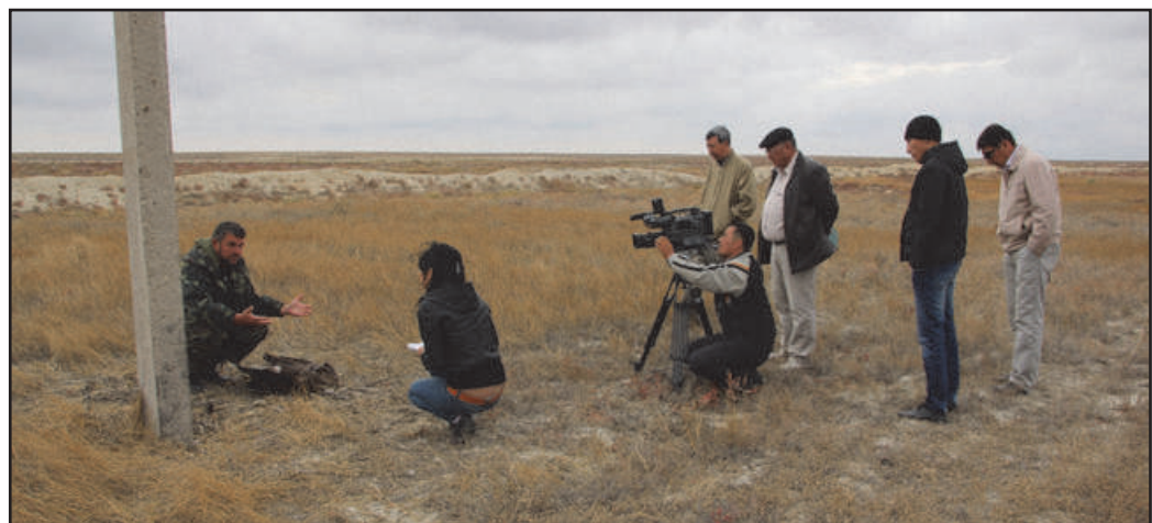
Examination of one of hazardous power lines near Atyrau with the TV crew of the “Ecological expedition “Eco – Atyrau” program. Photo by F. Saraev.
